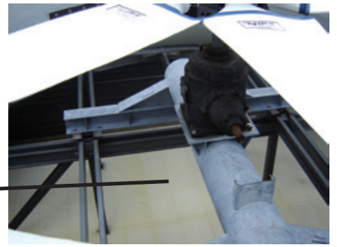
FM test cell with Franklin™ eliminators
