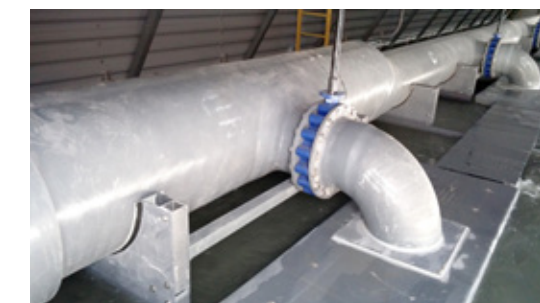
Fire-retardant water distribution system.
