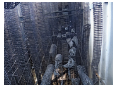
Following a successful Series ESX full-scale fire test there is minimal damage.
