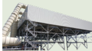
Air Cooled Steam Condenser
